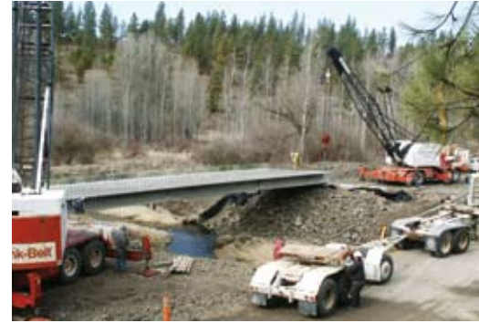
The Deep Creek Bridge uses thin-flange precast concrete deck bulb-tee girders with a cast-in-place concrete deck. It is the county's first with integral abutments.
