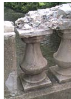
The original spindles were made using a mortar and were replaced with precast concrete spindles.
