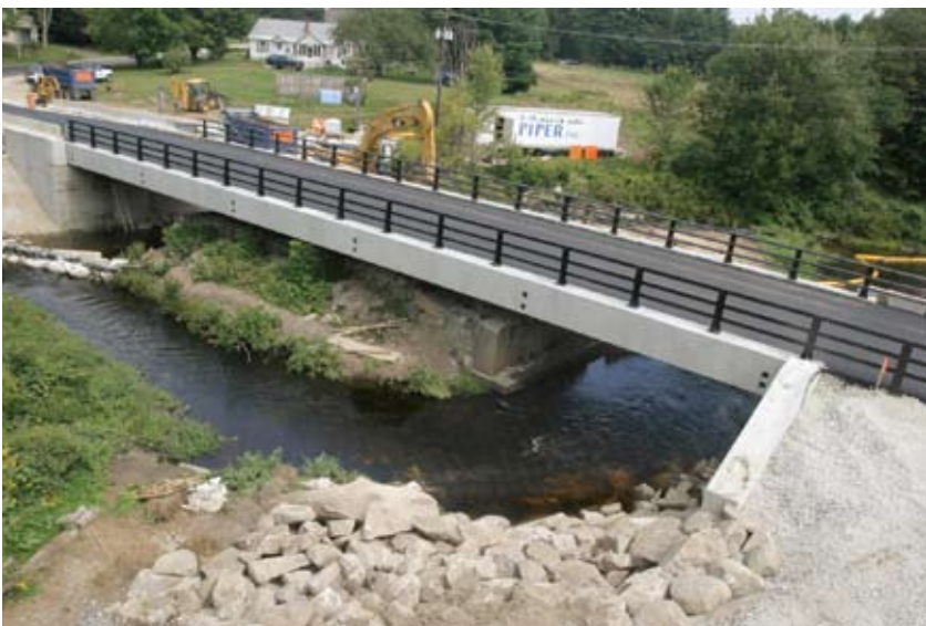
The new 115-foot, single-span precast concrete bridge carrying Mill Street over the Lamprey River in Epping, N.H., was finished with eight days of construction, which followed six weeks of preparation.
