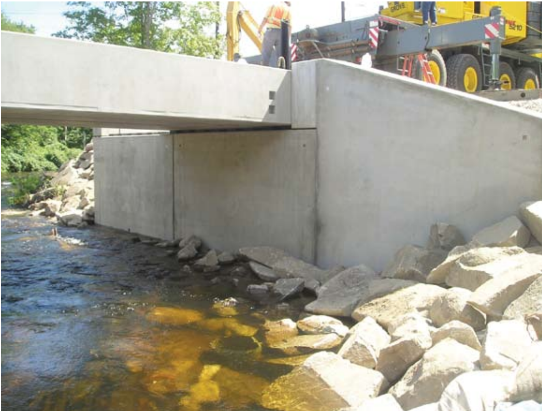
The bridge features a total precast concrete design, including box beams, abutments, wing walls and footings.
