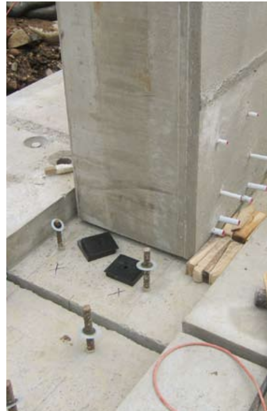
Precast concrete abutments were set onto the precast concrete footings using reinforcing bars grouted onto reinforcement extending from the footings.
