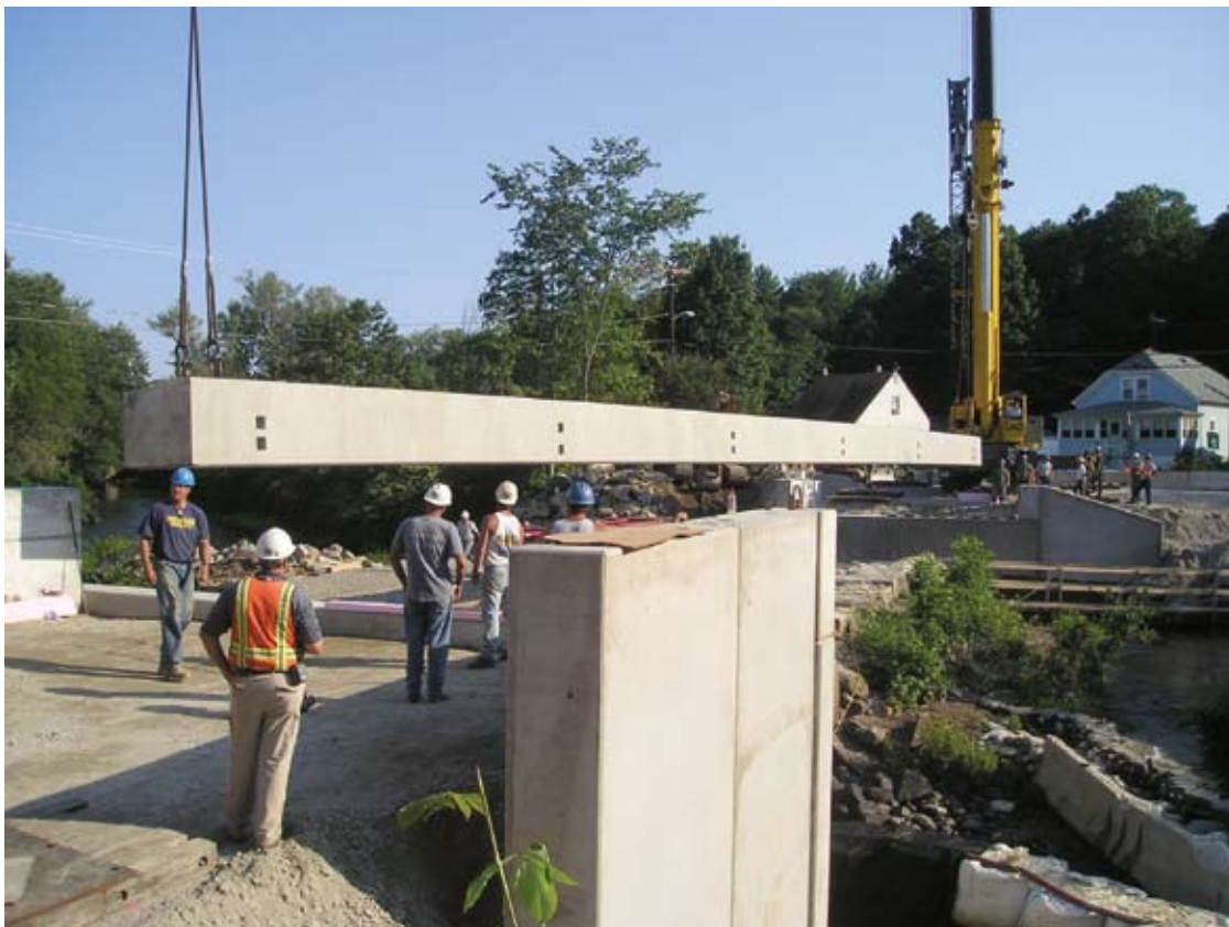
Seven precast concrete box beams were erected. They were cast with high-performance concrete, allowing the 115-foot bridge to be designed as a single span.
