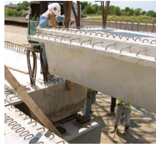
Pretopped U-Beams provide an instant work surface as illustrated in the bridge project, Loop 340 over I-35 in Waco, Texas.
