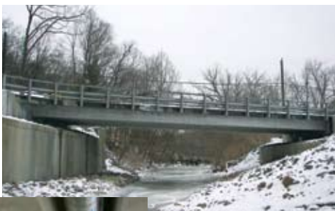
Spread box beams provide an economical solution for the new Zion Hill Bridge.
