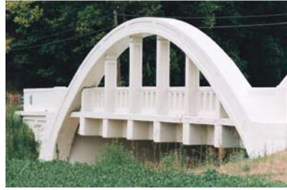
Willey Road Bridge in Hamilton County received the 1998 PCI Bridge Design Award for the Best Rehabilitated Bridge.
