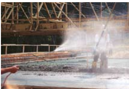
Fog misting can be used to reduce the evaporation rate.
