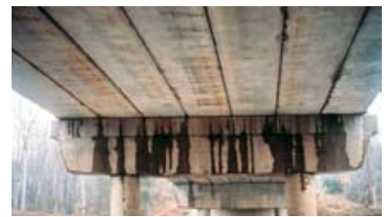
Leaking joints cause concrete deterioration and reinforcement corrosion.
