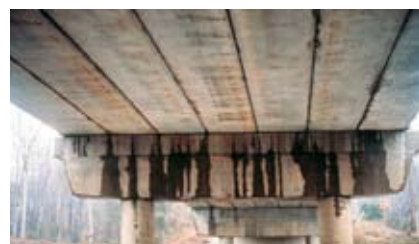
Leaking joints cause concrete deterioration and reinforcement corrosion.
