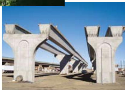
I-70 Trinidad Viaduct: NB 1985 ft long, SB 2058 ft long, 256-ft-long maximum span, 1000-ft-minimum radius.
