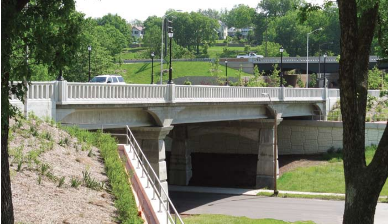
Aesthetic requirements played a key role in selecting the type of bridge for the 27th Street Bridge, Kansas City, Mo.
