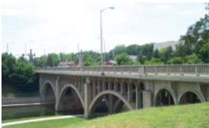
Rehabilitation of the Benton Boulevard Bridge in Kansas City, Mo., allowed preservation of an existing arch bridge originally constructed in 1923.
