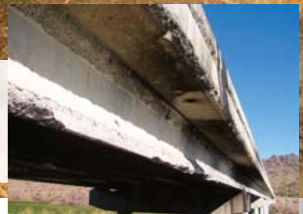
Following a fire on the Bill Williams River Bridge in Arizona, it was determined that the girders could be repaired. Photo: Arizona Department of Transportation.
