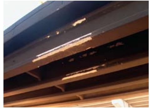
The blackened beams of the Bell Isle Bridge, Oklahoma City, Okla., were cleaned and the bridge was reopened. Photo: Oklahoma DOT.
