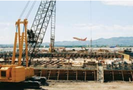
Deck concrete placement was carefully sequenced longitudinally and transversely. Photo: HDR Inc.
