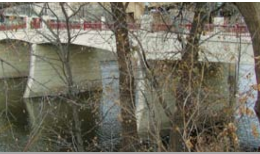
The Raspberry Island Bridge features five spans of cast-in-place concrete slab girders. The bridge ties in with the nearby Harriett Island trail system and the River Walk, and features "St. Paul Rail" designed hand rails.
