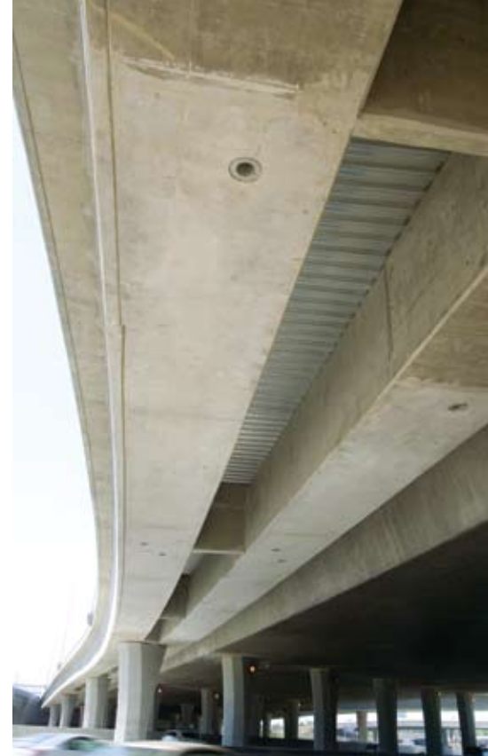
Curved precast, prestressed concrete spliced girders span I-5 at the interchange with State Route 22.
