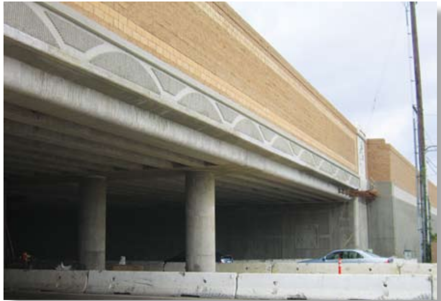
Completed low-profile precast concrete girder undercrossing on SR 22. Photo: Vinh Trinh, PBS&J.
