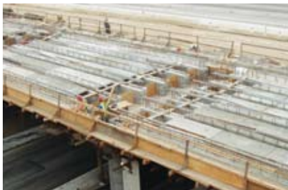
Formwork is placed around precast girders in the construction of a seismic-resistant integral connection with the columns. Photo: Jay Holombo, PBS&J.
