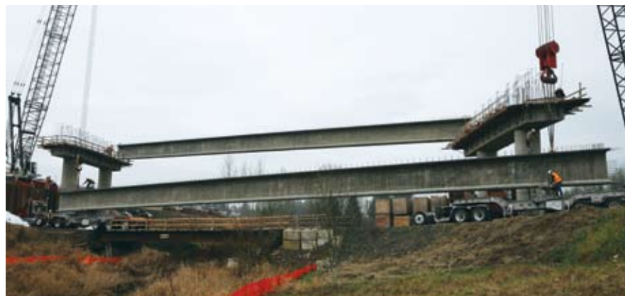
The SR 502 bridge over I-5 near Vancouver uses W83Gs with a girder length of 176 ft.
