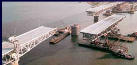
George P. Coleman Memorial Bridge - Virginia Lightweight concrete deck on widened replacement trusses.
