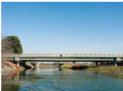
The Daggett Road Bridge environmental constraints played a key role in determining the type of bridge. Photo: DMJM Harris.
