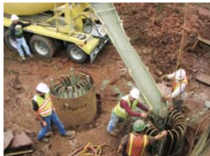
Self-consolidating concrete was used in the drilled shafts of the Route 28 Bridge over Broad Run.
