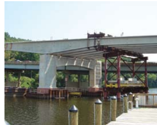
The first spliced beams were used on Route 123 Bridge over the Occoquan River.
