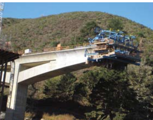
Form travelers are used to construct the main span cast-in-place segments over the environmentally sensitive valley below.
