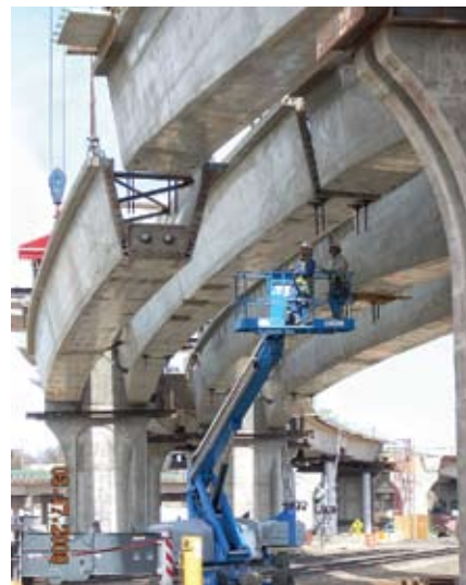
As precast products evolve into more-complex systems, the demands for quality assurance increase accordingly. (Photo: Summit Engineering Group Inc., Littleton, Colo.)
