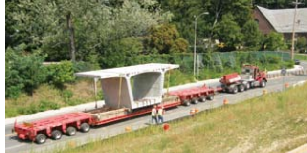
To protect the waterway near the site, precast concrete segments were barged from the precaster's plant in Cape Charles, Va., to a location several miles from the project and then hauled by specialized trailers to the site.
