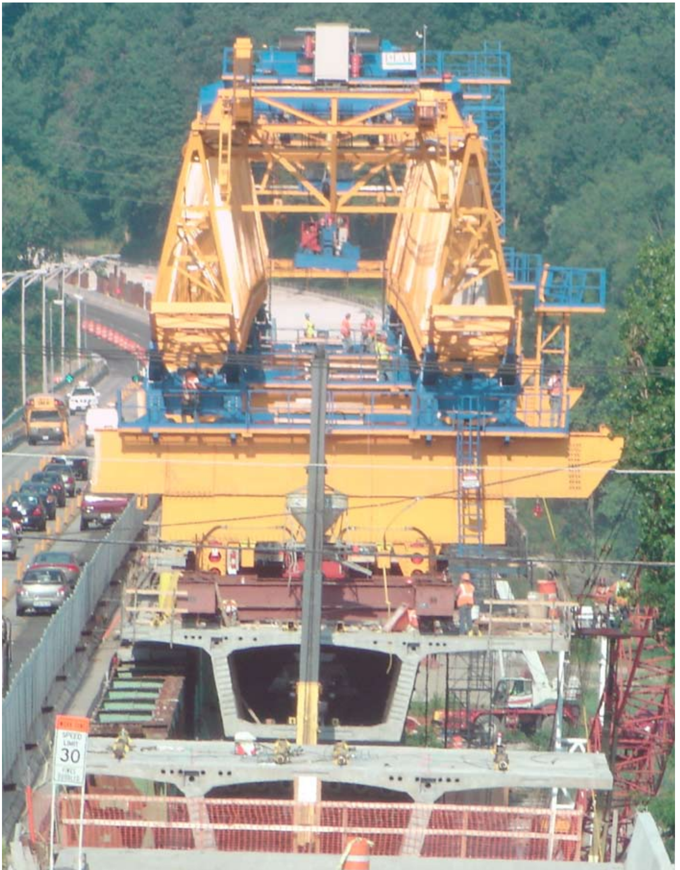
Concrete is placed at the closure pour at pier 7 using a crane and bucket while the gantry is positioned at piers 6 and 7. In the foreground are the pier 8 pier table and the east abutment. Photo: Rich Lorenzen.
