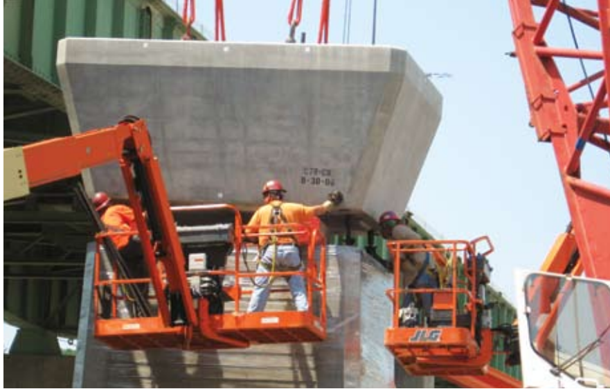
Ironworkers align the couplers for the post tensioning bars as they set the precast concrete column cap segment at pier 7. Photo: Renata Magoc.
