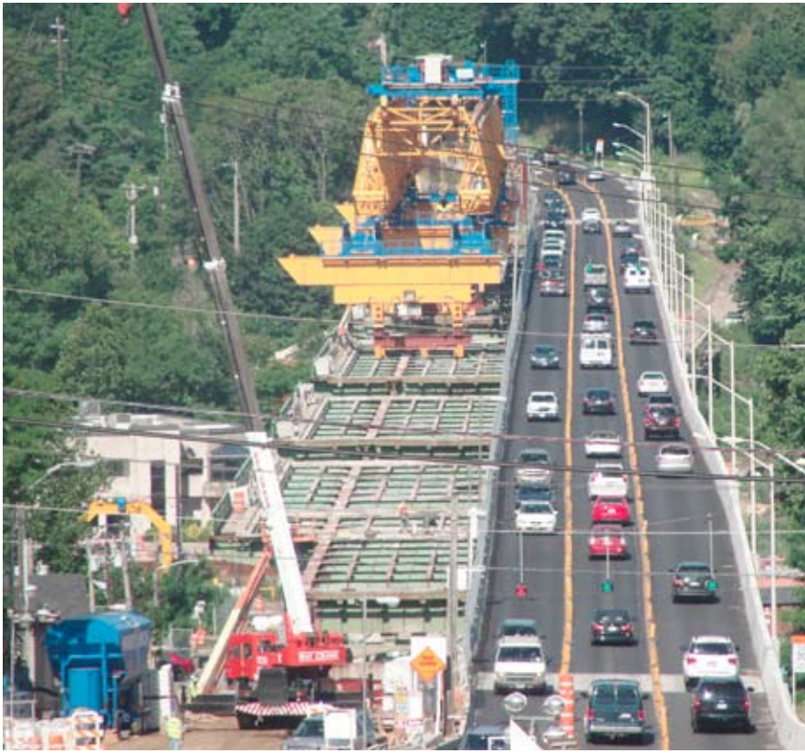
After the north side of the bridge was constructed, the gantry crane was shifted to the south to remove the steel frame of the existing bridge. Photo: Rich Lorenzen.
