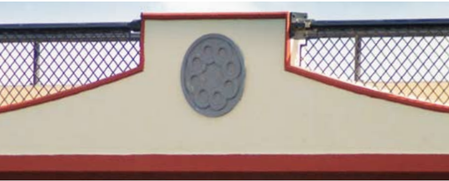
The 40 th Street Bridge in Tampa, Fla., features a single post-tensioned concrete span with special aesthetic treatments created by local high-school art students. They learned the basics of conceptual design, and contest winners had their designs' ideas, colors, and shapes incorporated into the formal aesthetic plan.
