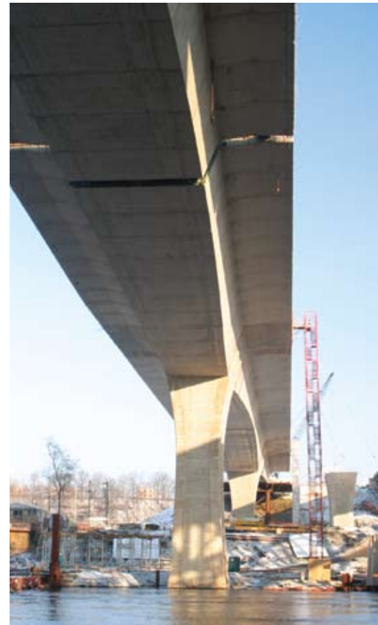
A 4-ft closure is all that remains to complete a 380 ft span at a height of 100 ft over the Allegheny River. All photos: © FIGG.
