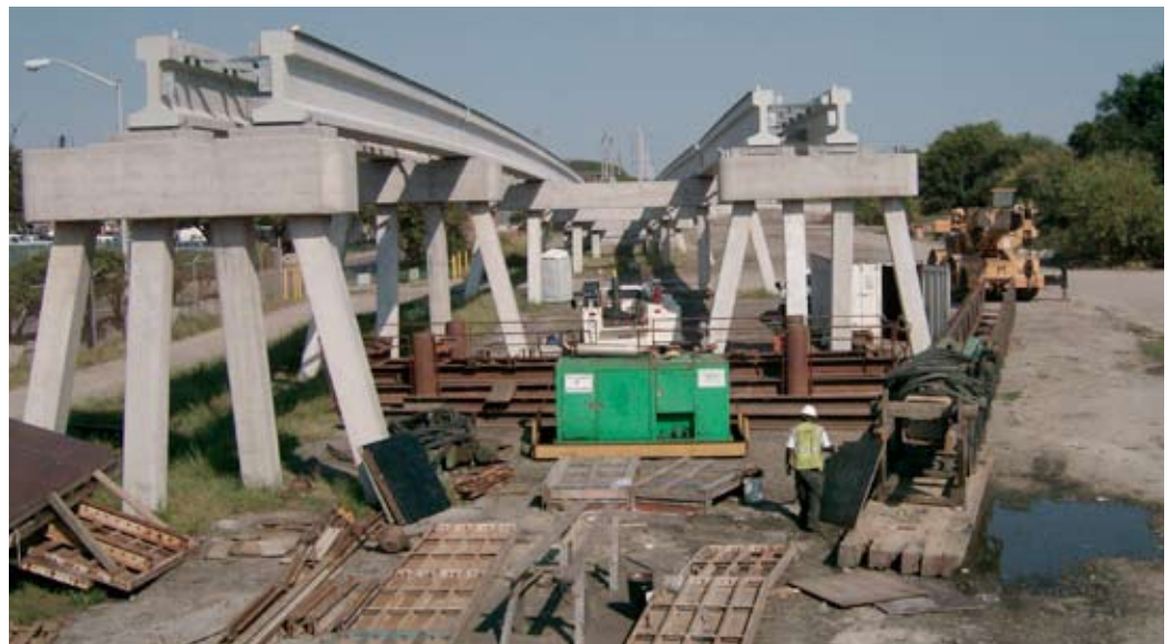
Separate single track open deck spans, looking east from bent 38. Photo courtesy of Bryant Contracting.
