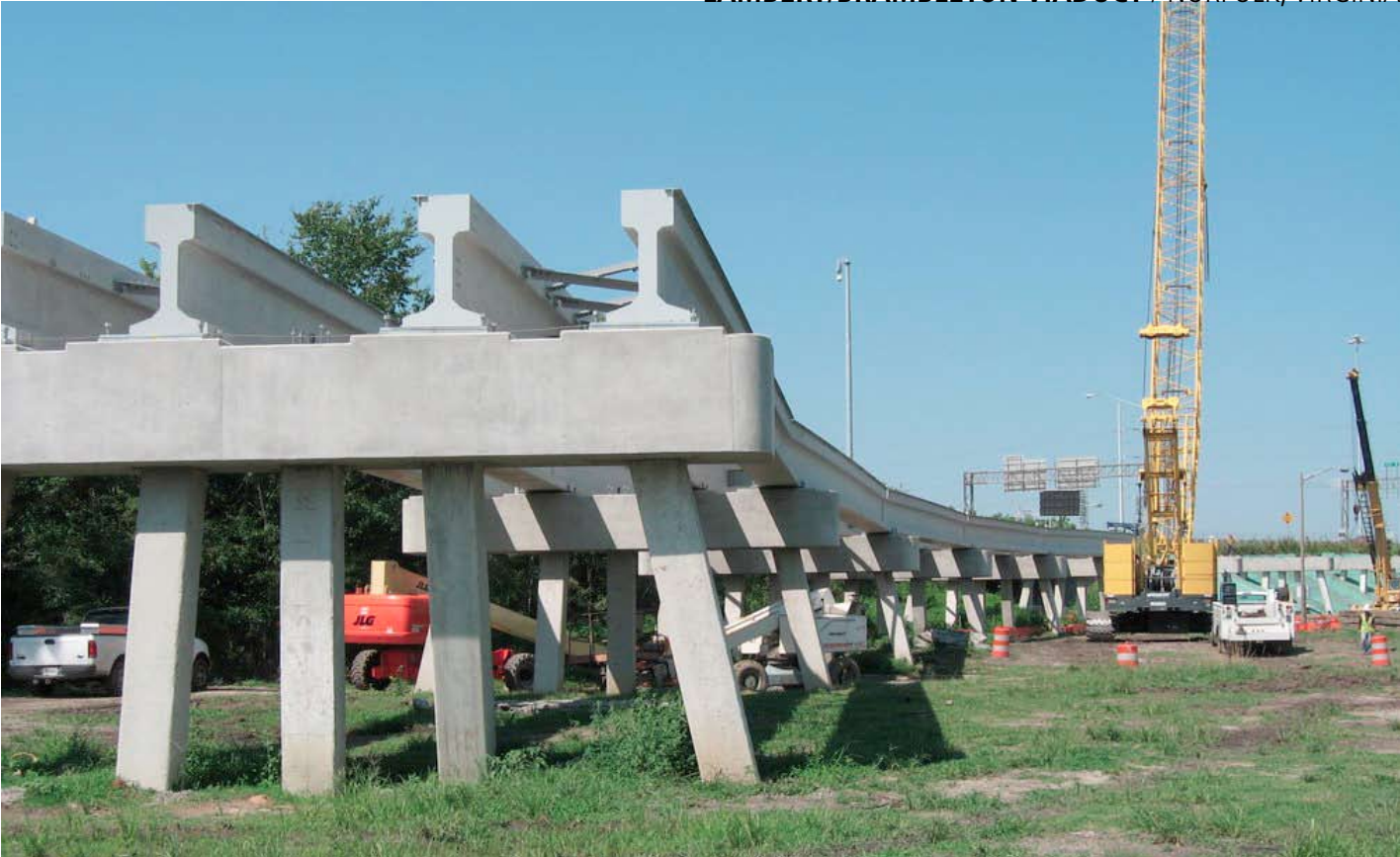
General view of the aerial structure looking west at a typical pile bent and the open deck spans. The embedded WT steel section can be seen in the outside edges of two of the girders. Photo courtesy of HRT.
