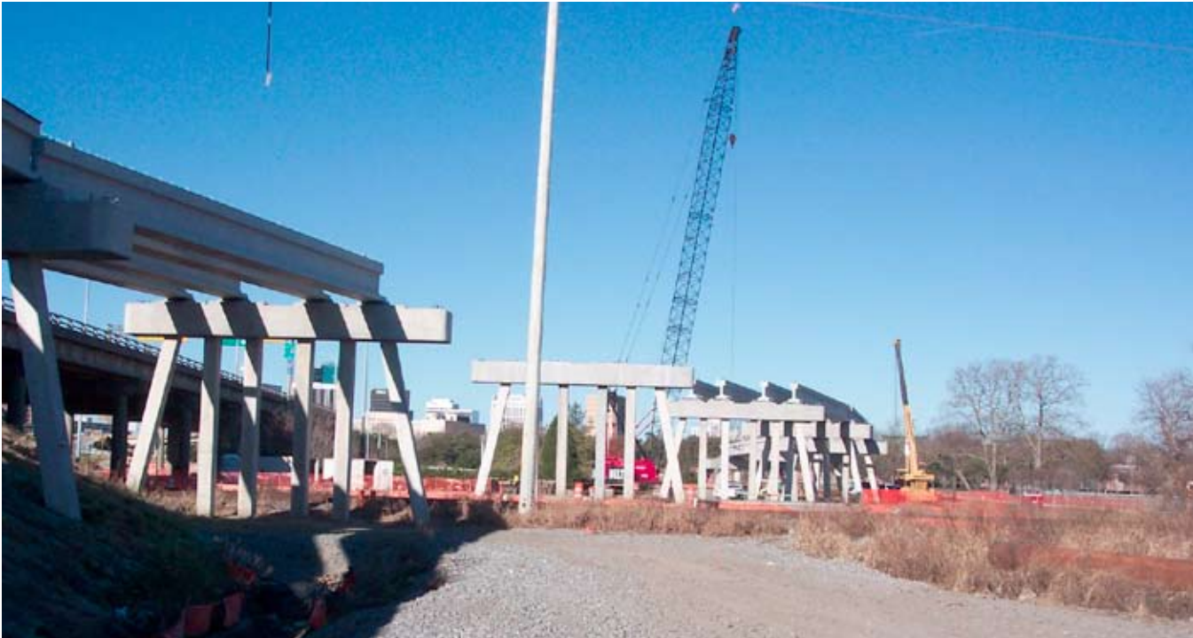
Construction of the spans over Lamberts Point Branch Line. Photo courtesy of PB.
