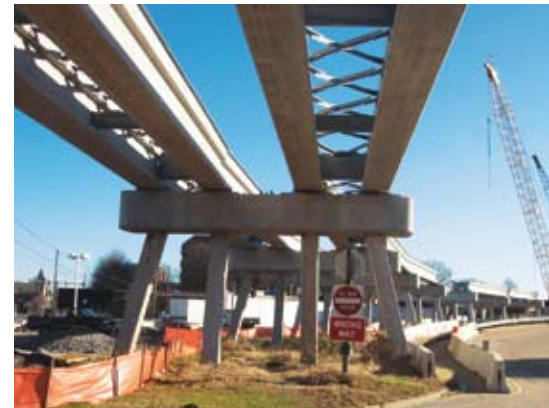
Lateral bracing and diaphragms in typical open deck span. Photo: PB Americas.
