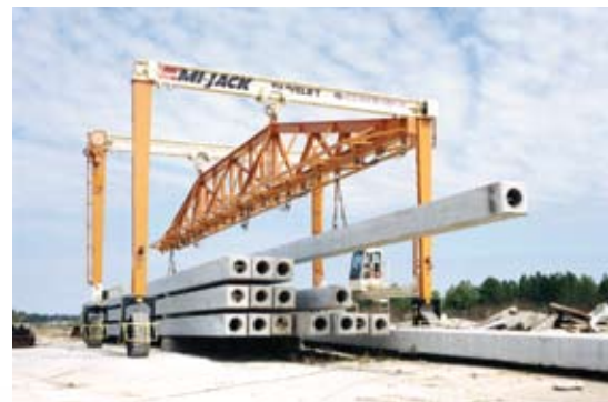
Twenty-four-inch- and 30-in.-square piles were cast with high-strength concrete permitting longer individual lengths.
