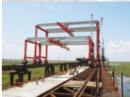
The new bridge on the LA 1 Highway is being constructed from the top down to minimize impact on the coastal wetlands areas over which the bridge is being constructed.
