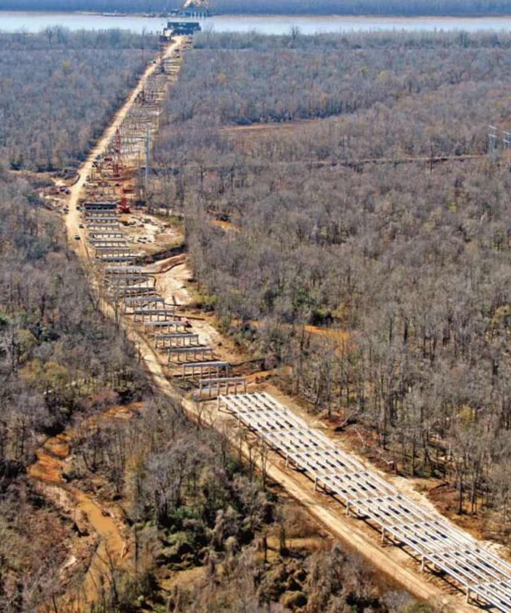
The 2.44-mile-long John James Audubon Bridge crossing the Mississippi River, to be completed in late 2010, will be the longest cable-stayed bridge in North America. In addition to the precast concrete structure, the project involves seven other bridges featuring Type III AASHTO precast, prestressed concrete girders and 72-in.-deep bulb-tee girders with cast-in-place decks.
