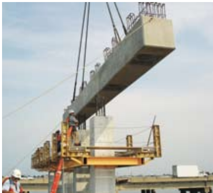
A precast concrete bent cap being set on precast concrete piles for the I-10 Twin Spans Bridges over Lake Pontchartrain.
