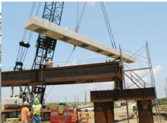
Nine miles of the LA 1 Highway Bridge are currently being constructed, while an additional 9 miles are being planned and designed. Here a precast concrete pile bent cap is being moved into position for installation.
