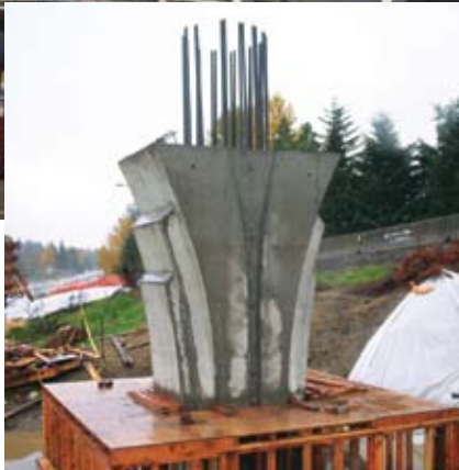
Cast-in-place columns were built for the intermediate piers, using designs influenced by the state's new Context-Sensitive Solution guidelines.
