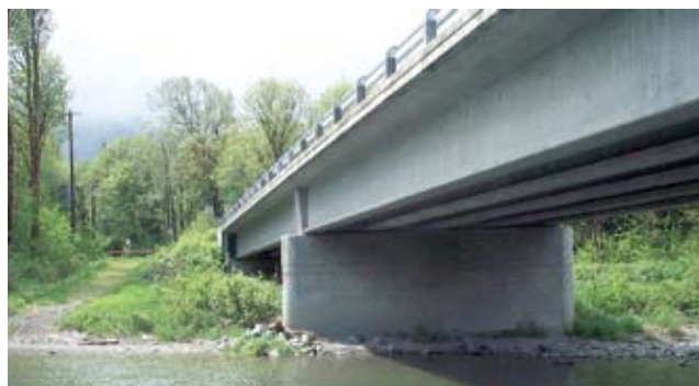
North Fork Stillaguamish River Bridge 424. Nearly 95% of the county bridges cross water, and virtually all of those waterways impact endangered species.
