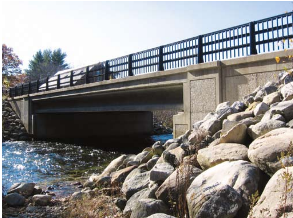
Completed Bristol Bridge carrying NH 3A over the Newfound River used partial-depth deck panels.
