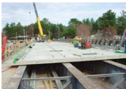
NHDOT's first use of precast, prestressed full-depth deck panels on the redecking of the Mosquito Bridge over Lake Winnisquam.
