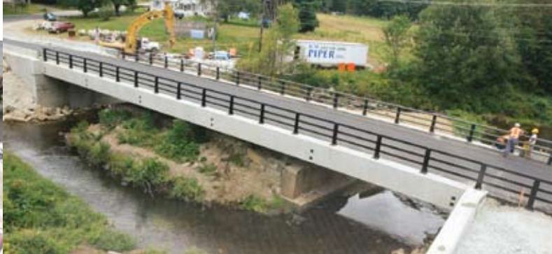
Eight days after the first precast footing piece was placed, the Mill Street Bridge in Epping was paved and opened to traffic.
