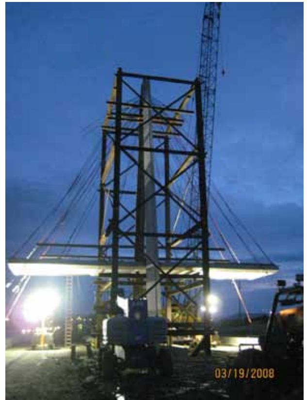
The nighttime erection of precast concrete deck panels. Photo: OBEC Consulting Engineers.
