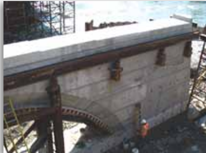
The completed half-pier showing temporary supports under the arch and beam that will be used to support steel stringers that in turn support concrete forms.
