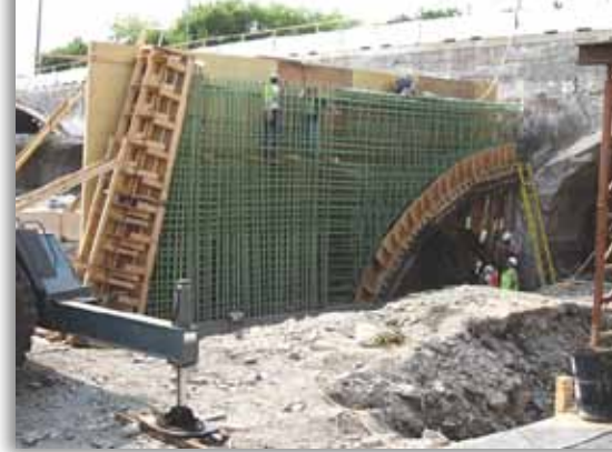
With half of the original structure demolished, construction begins on the first half-pier.
