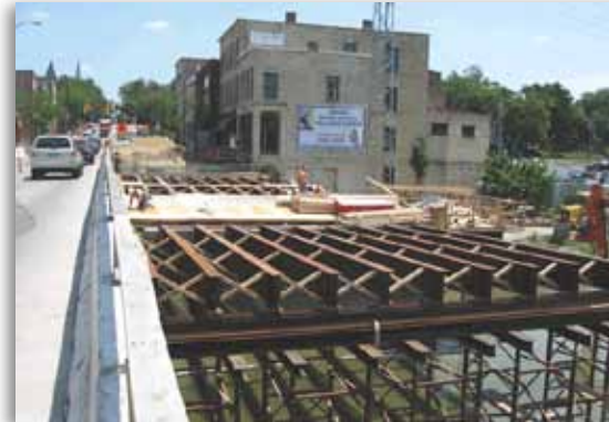
Falsework is shown in the river to support stringers and deck formwork.
