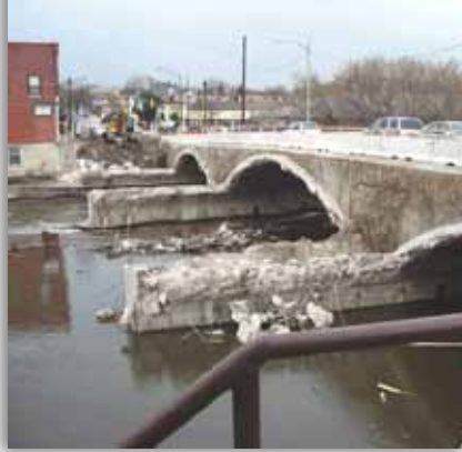
Demolition of one-half of original structure is nearly complete. A temporary soil retention wall was used to retain the soil in the earth-filled arches. All construction photos: AECOM.
