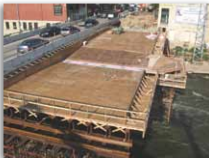
Forms shown completed for approximately one-half of the first stage of construction. Note the forming of the soffit of the first of four river outlooks.
