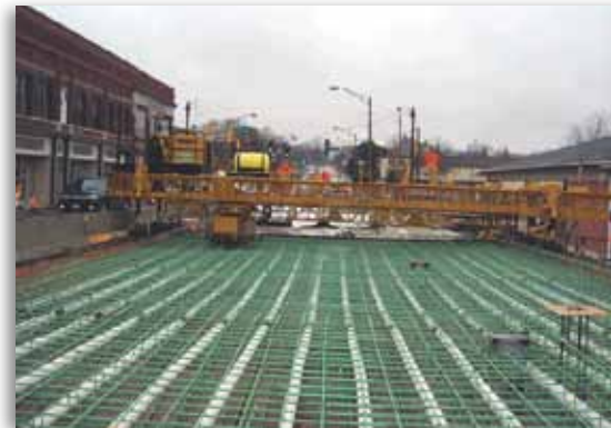
Concrete placement is ready to proceed during the first stage of construction.
