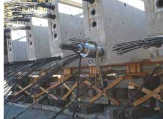
The first stage post-tensioning was done in the staging area. The bottom tendons needed to be stressed simultaneously from opposite ends of the girder to prevent eccentricity.
