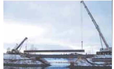
The Crescent Bar Bridge over the Columbia River is a 130-ft-long, single-span, prestressed concrete deck bulb-tee bridge shown here during girder placement. Photo: Jeff Tincher, Grant County.
