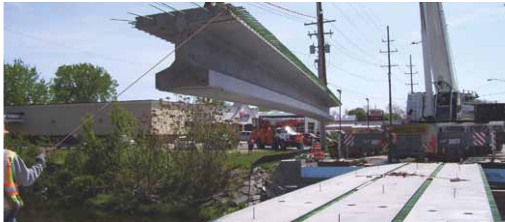
UHPC was used to connect these deck bulb tees in the Route 31 Bridge over Canandaigua Outlet in the Village of Lyons, N.Y. Tests showed that the No. 6 epoxy-coated reinforcement was fully developed with a 6-in. lap in the joint. 2 Photo: New York State Department of Transportation.
