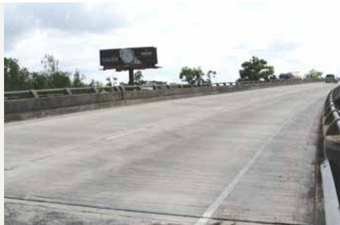
A 3-in.-thick concrete overlay was applied to this six-span bridge under the LADOTD preventative maintenance program.
