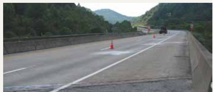
Bridge with lane closed to perform a deck condition survey. All Photos: Wiss, Janney, Elstner Associates Inc.
