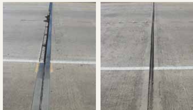
This is a failed steel armored expansion joint that was eligible for repair, and the joint following rehabilitation with polymer concrete.
