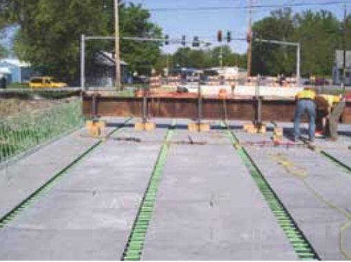
Adjacent deck bulb tees being aligned for level prior to field-casting a UHPC longitudinal joint on the State Route 31 Bridge over the Canandigua Outlet in Lyons, N.Y. Photo: New York State DOT.
