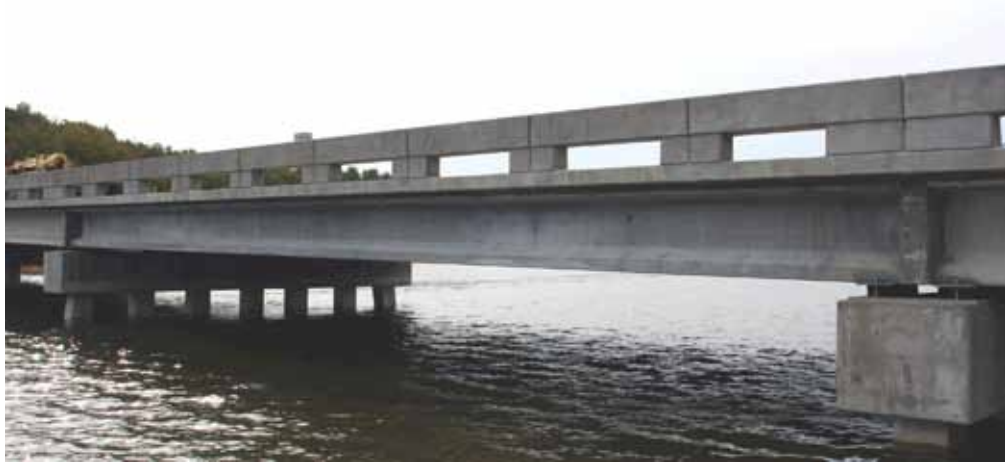
The Cat Point Creek Bridge near Warsaw, Va., uses standard VDOT bulb-tee UHPC girders, 45 in. deep, spanning 85 ft. Photo: FHWA.
