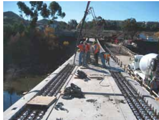
Concrete is placed in the longitudinal trough that was cast in the panels.
