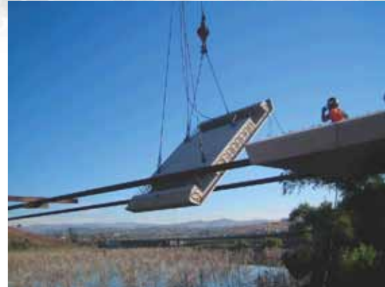
One of 87 precast concrete panels is shown during the typical erection procedure.
