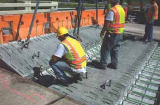
A precast concrete section being lowered into place adjacent to another during the rehabilitation of Bridge 6679.
