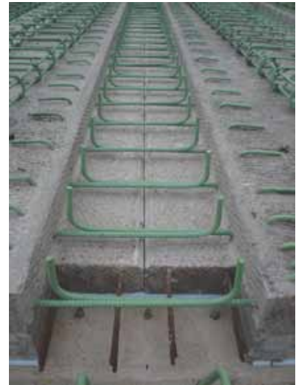
View of a longitudinal joint between precast sections before installing field-placed reinforcement.
