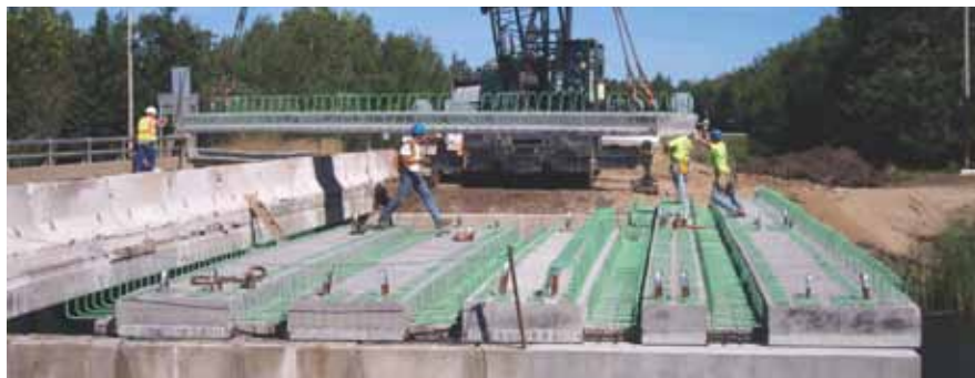
On Bridge 04002, a precast concrete beam is being moved into place alongside five sections that have already been erected. The typical 6 ft 0 in. beam width can be changed to accommodate bridge width.
