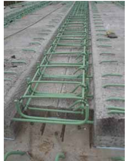
View of a longitudinal joint after the placement of the “drop-in” reinforcing cage.
