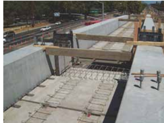
The grade-separation structure features a "trough" cross-section, consisting of three precast, prestressed concrete through-girders spanning in the longitudinal direction, and precast, prestressed concrete slabs spanning between adjacent girders in the transverse direction.
