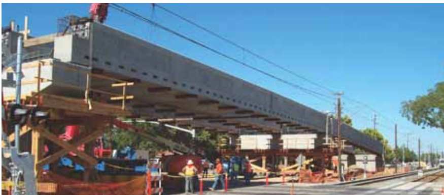
The difficulty of constructing a grade separation in close proximity to operating light-rail and freight tracks created significant complexities.
