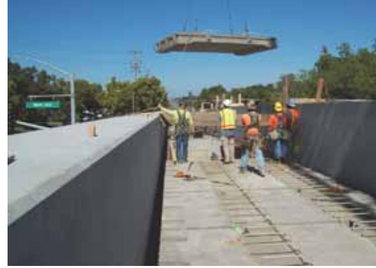
Installation of the precast concrete deck slabs took place during normal working hours.
