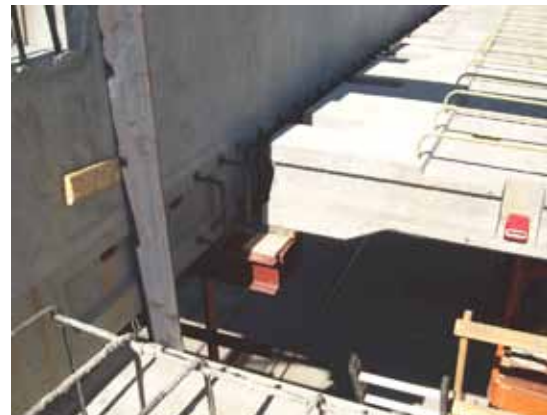
After erection, the deck-slab panels were connected with cast-in-place concrete closure strips and longitudinal post-tensioning. They are integrated into the superstructure by post-tensioning transverse tendons, which also pass through the girders and longitudinal closure pours.
