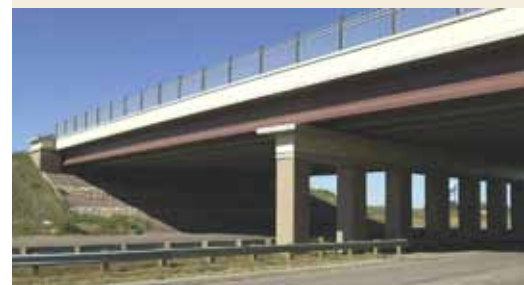
The inspiration for articulation and coloring of the concrete elements of this two-span bridge, First Street over I-29 near Sergeant Bluff, came from nearby examples of Prairie School architecture.
