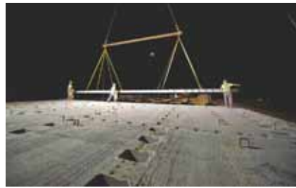
Full-width deck panel placement at the 24th Street project site in Council Bluffs, the first Highways for LIFE project in Iowa.
