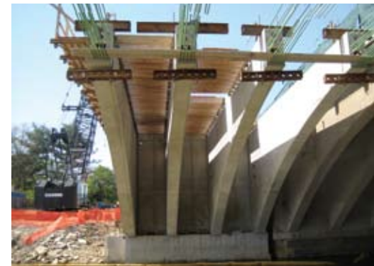
Formwork being constructed for the cast-in-place concrete deck placement. Photo: Cianbro Corp.
