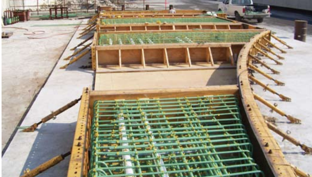
Because the precast concrete arches required a depth of 20 ft, they were cast horizontally, with all seven segments for each half-arch cast in one setup. Photo: Northeast Prestressed Products LLC.
