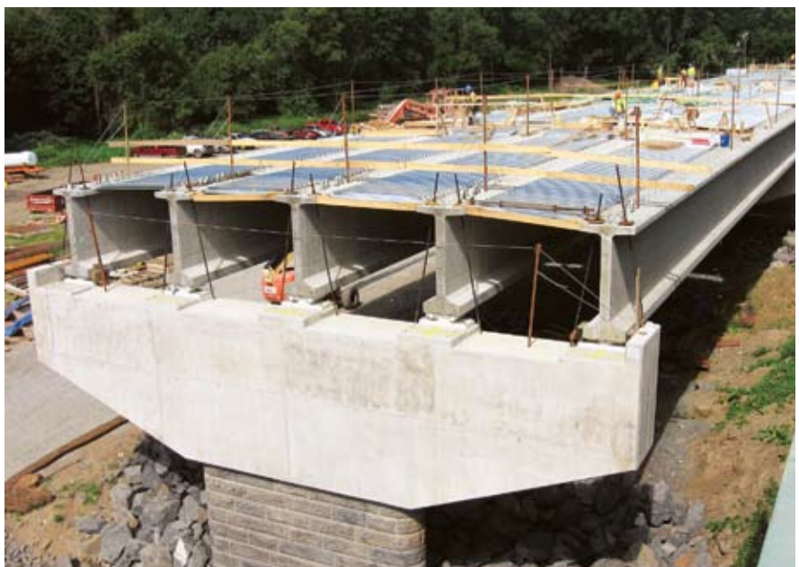
The 1319-ft-long 8th Street Bridge in Luzerne County, Pa., will feature 10 spans of precast, prestressed concrete bulb-tee girders. The project, to open summer 2010, replaces a deteriorated structure on the site.
