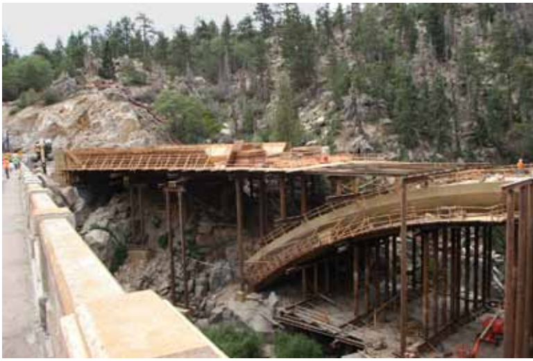
All but the bottom form for the arches have been removed while forming begins for the box girder.
