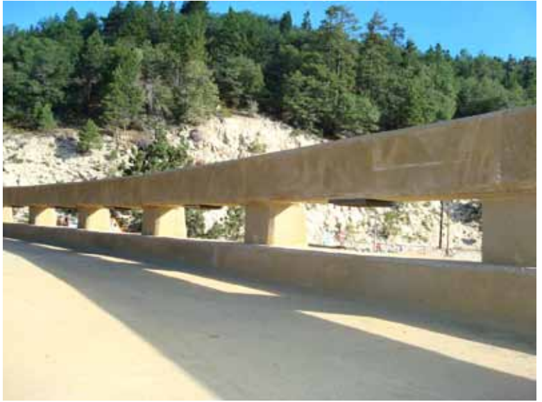
A special open concrete barrier affords views of the dam to the north and the ravine to the south.
