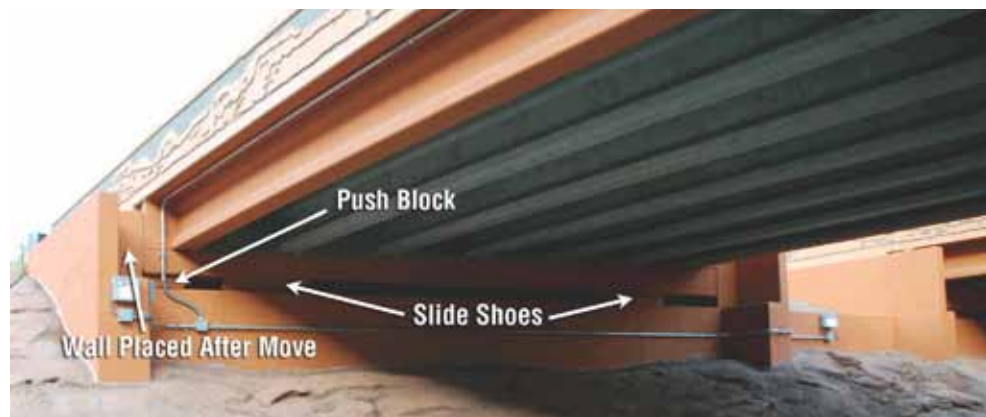
New westbound structure in place and complete. The push block and slide shoes can be seen.
