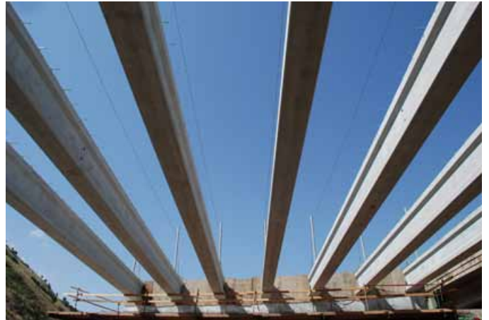
I-80 at Echo Dam Road Bridge is constructed of 80-ft-long AASHTO Type II precast, prestressed concrete beams.
