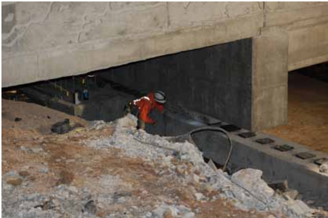
A workman monitors the slide operation to make sure the slide shoe moves cleanly onto the PTFE-coated bearing pads.
