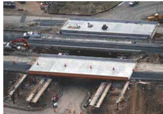
The westbound bridge is in place as crews prepare for partial demolition of the eastbound bridge.
