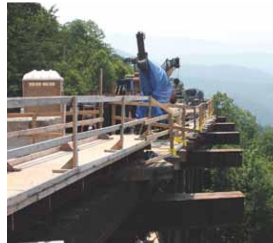
On the project site, a temporary trestle is in place as work gets started on Foothills Parkway Bridge No. 2. Photo: FHWA.
