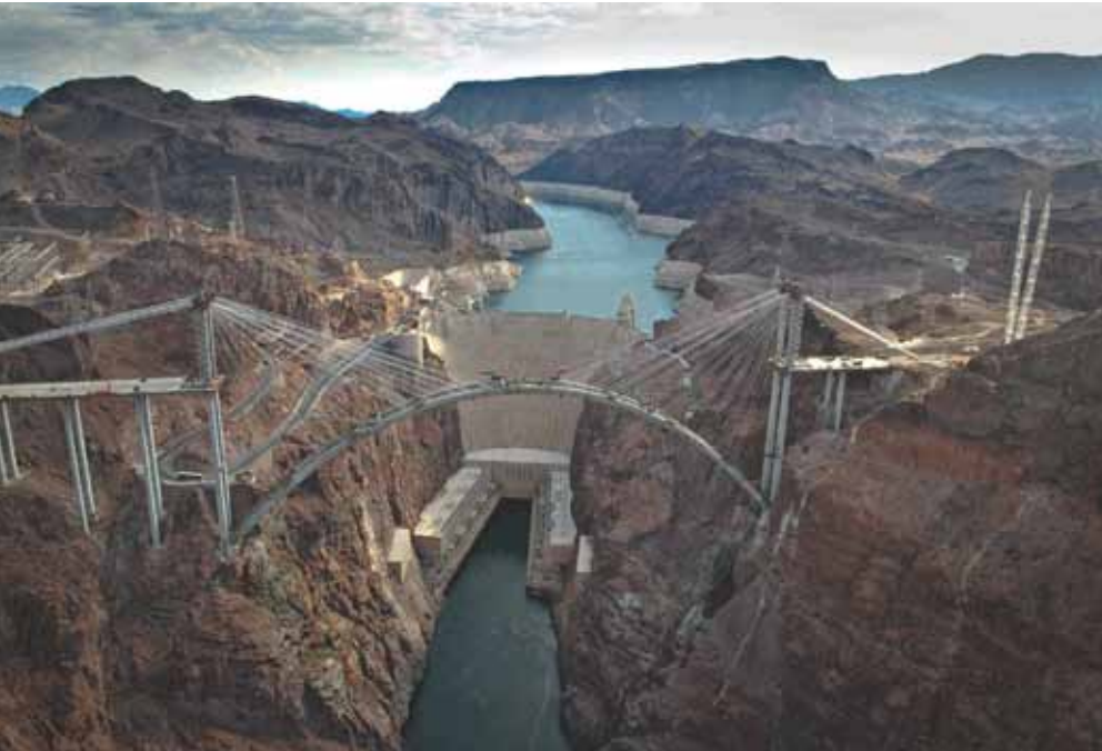
McNary Bergeron provided construction engineering for the cast-in-place arch structure and temporary stay-cable system used to support the Hoover Dam Bypass Colorado River Bridge. It was one of the first high-profile projects for the company, which was founded in 2003. All photos: McNary Bergeron & Associates Inc.
