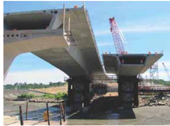
By designing Veterans Memorial Bridge Replacement in Portland, Maine, in a similar style to the earlier Route 36 Highlands Bridge in New Jersey, McNary Bergeron allowed the precaster, who was the same for both projects, to reuse the original forms, saving costs.
