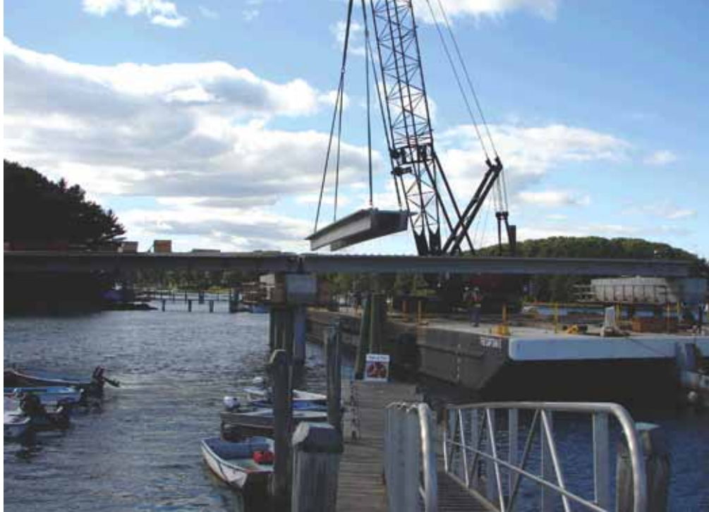
Route 103 over the York River in Maine employs the Northeast Extreme Tee (NEXT) Beam, developed by the Northeast Chapter of PCI to accommodate accelerated construction of bridges in the region. (Additional information on the NEXT beam and York River Bridge can be found on page 46 in this issue.) Photo: Dailey Precast LLC.
