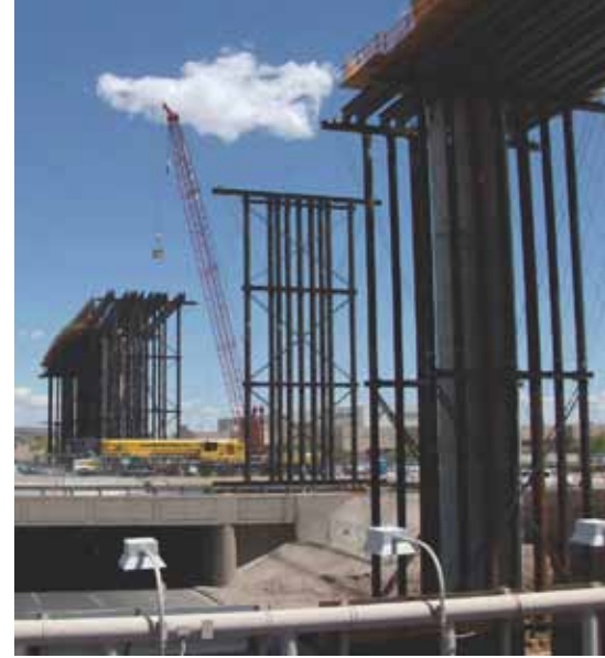
The erection of falsework for the center span showing the proximity of Sky Harbor Boulevard crossing under Taxiway "R." Photo: Gannett Fleming Inc.
