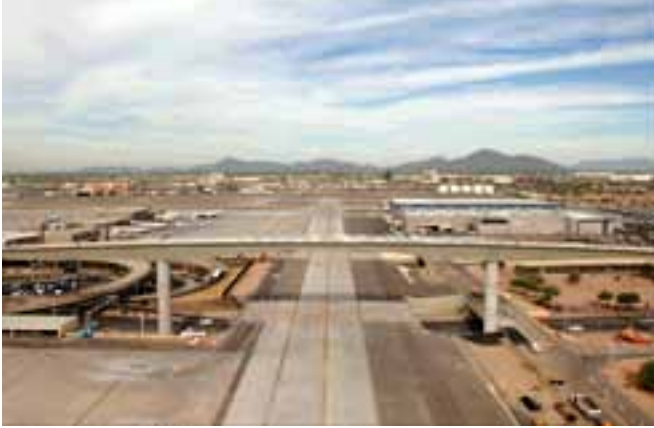
Taxiway "R" looking north with falsework removed and barrier placed on center span. Photo Rights: Hensel Phelps Construction Co.; Photo Credit: Visions in Photography.
