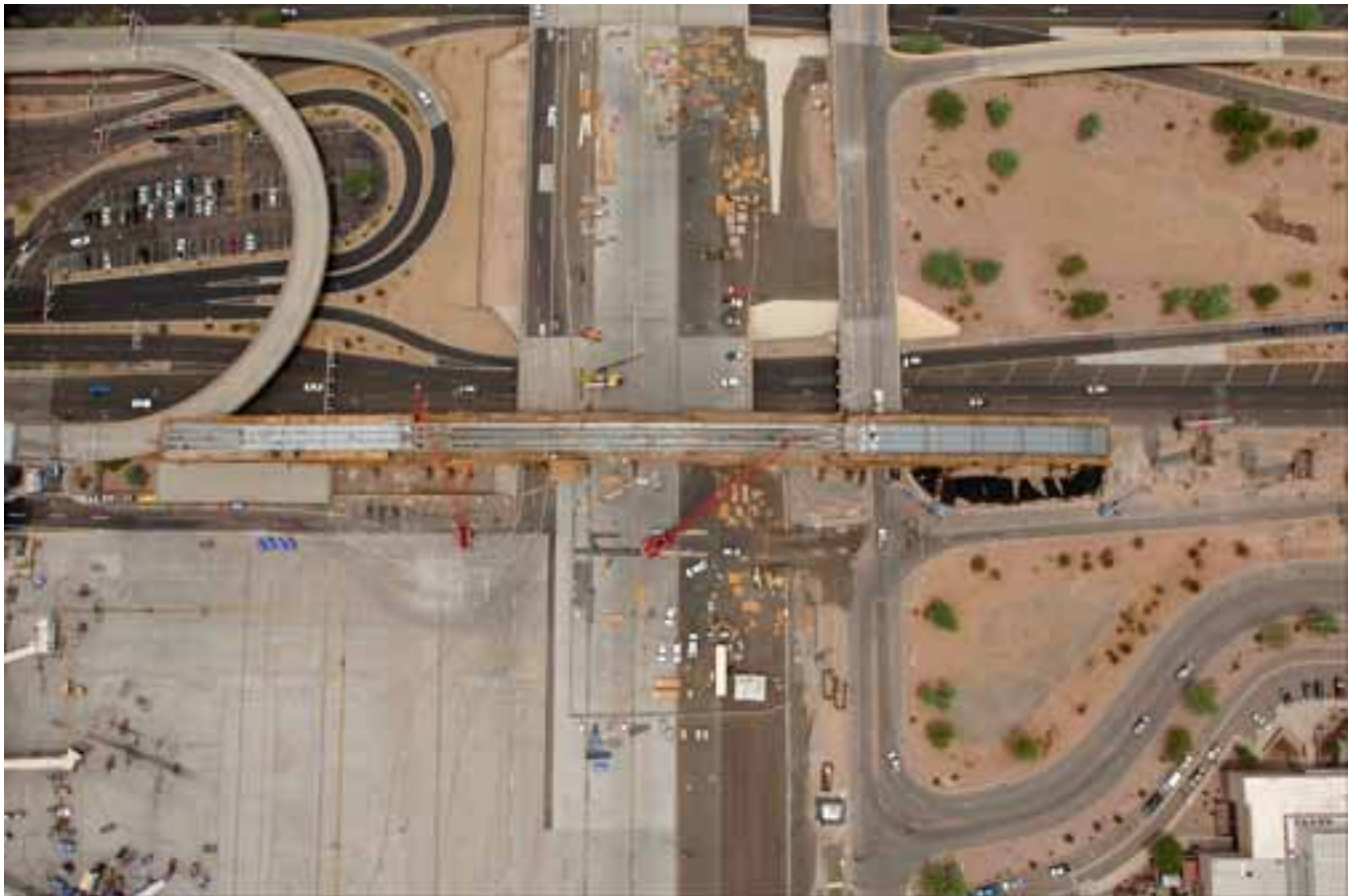
Aerial view of Taxiway "R" with box girder floor and webs complete and the deck being formed. Photo Rights: Hensel Phelps Construction Co.; Photo Credit: Visions in Photography.
