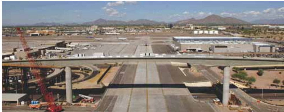
Taxiway "R" looking north showing removal of end span falsework. Photo Rights: Hensel Phelps Construction Co.; Photo Credit: Visions in Photography.
