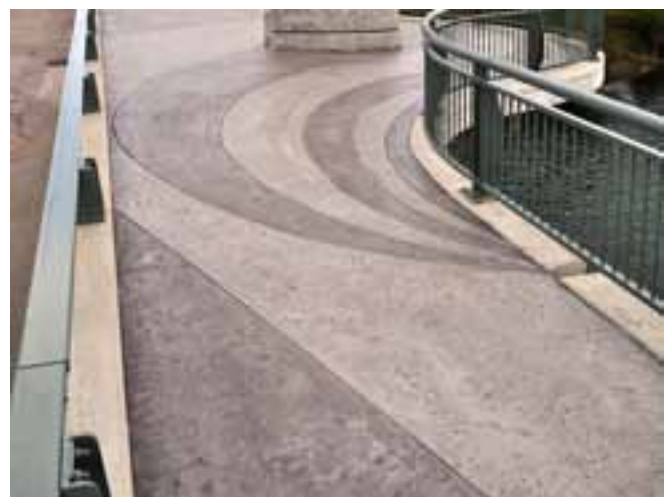
Pigmented and stamped concrete overlays on sidewalks add to the aesthetics of the overlooks. Photo: C. Hodge, T.Y. Lin International.
