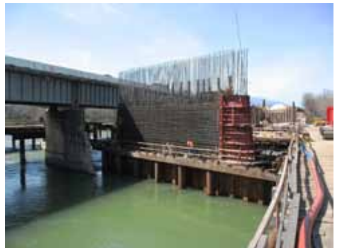
Stage 2 construction of pier wall with steel end form to create architectural shape. Photo: K. Pope, T.Y. Lin International.
