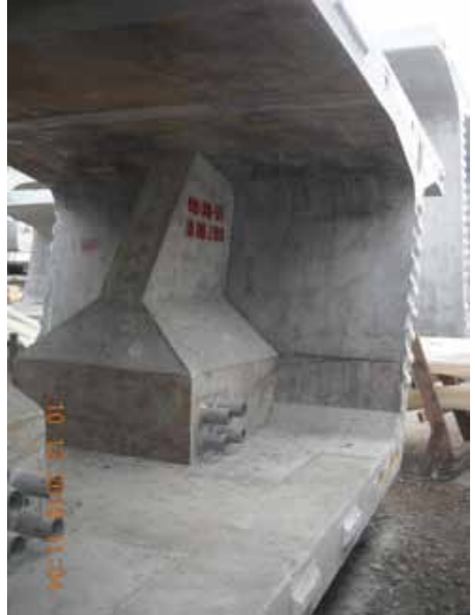
A segment with full-height intermediate deviator diaphragms. Photo: Rizzani de Eccher USA.
