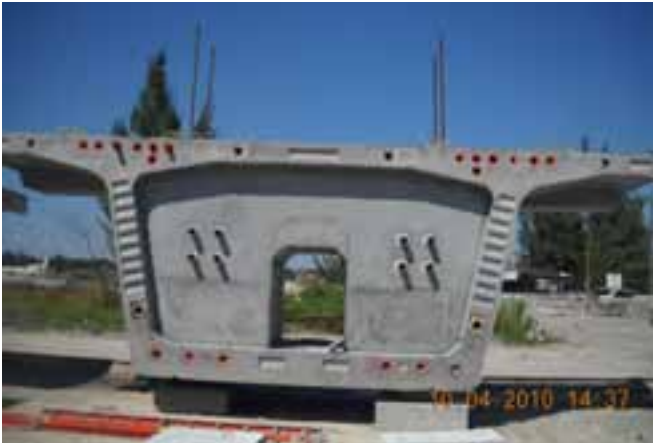
A dual-track pier diaphragm segment as used on single piers. Photo: URS Corporation.
