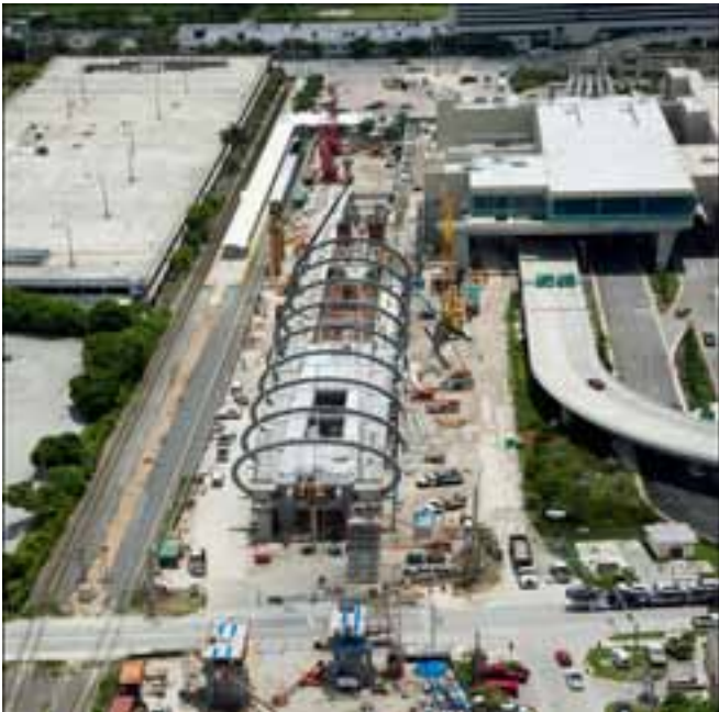
Aerial view of the Miami Intermodal Center (MIC) station during construction. Photo: URS Corporation.
