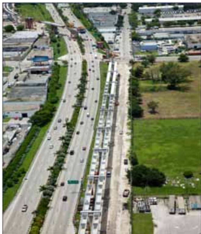
In this section of the Miami Intermodal Center—Earlington Heights Connector, 72-in.-deep Florida U-beams parallel to SR 112 were used. Photo: URS Corporation.
