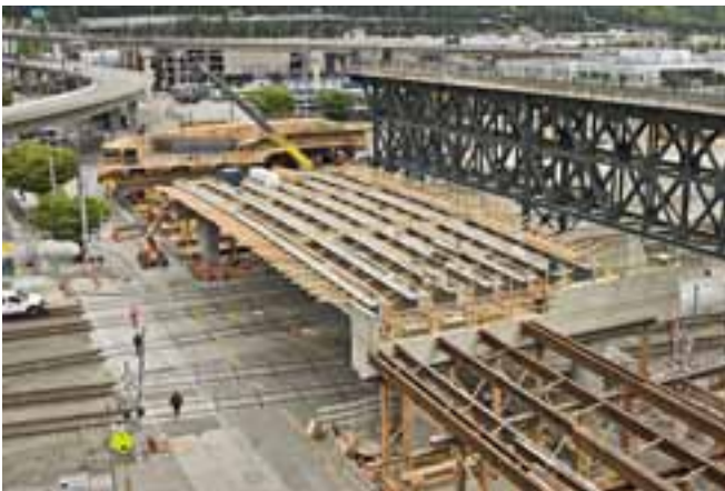
The precast, prestressed, precambered concrete I-beams have been set over the railroad tracks. Photo: Washington State Department of Transportation.
