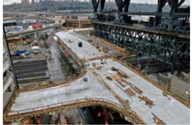
The roadway of the Royal Brougham Bridge had to be high enough to cross over the trains, yet low enough to allow entry to the second level of the parking garage via the short horizontal roadway segment in the foreground. Photo: Washington State Department of Transportation.
