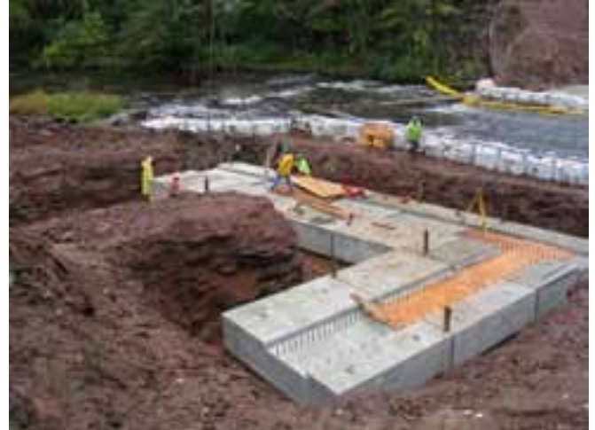
The precast concrete footings were set and aligned with plywood templates to ensure fit-up of the walls over the dowel bars. Photo: Arborio Corporation.
