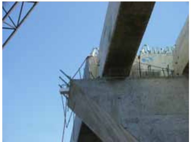
Precast solid and box beams sit atop the transverse cast-in-place concrete transfer/tie beam. Photo: Woolpert Inc.
