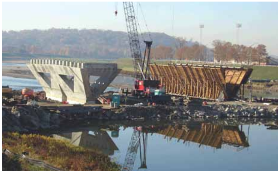
Legs of the Y-shaped piers are tied transversely with cast-in-place concrete box girders and longitudinally with precast concrete solid beams.
