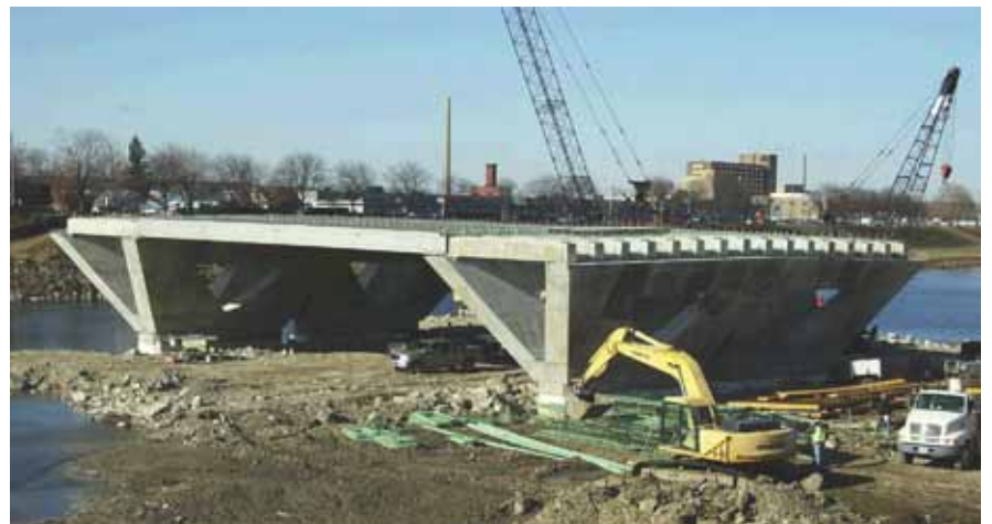
Solid, 42-in.-deep, precast concrete beams tie the legs of the Y-shaped piers and butt against the ends of 48-in.-deep, precast, prestressed concrete box beams spanning from pier to pier.
