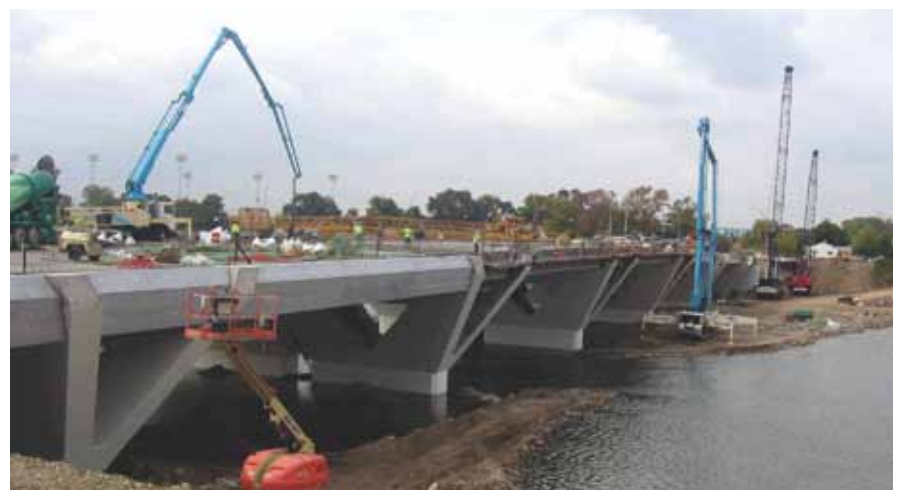
The dramatic effects of the precast concrete fascia panels can be seen during their installation.
